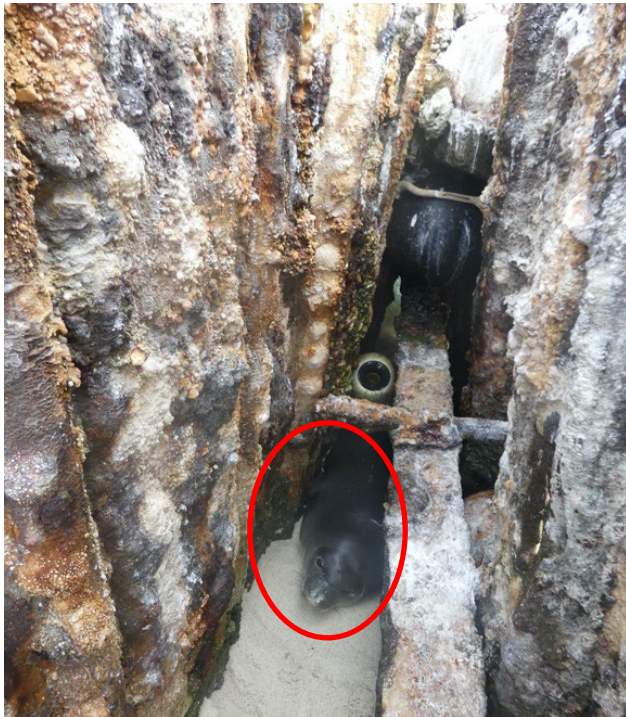
Monk seal pup (red circle) trapped and pinned inside a Tern Wall seawall. The pup was rescued with great difficulty as the tide was rising, and was ultimately saved from drowning (NOAA).
